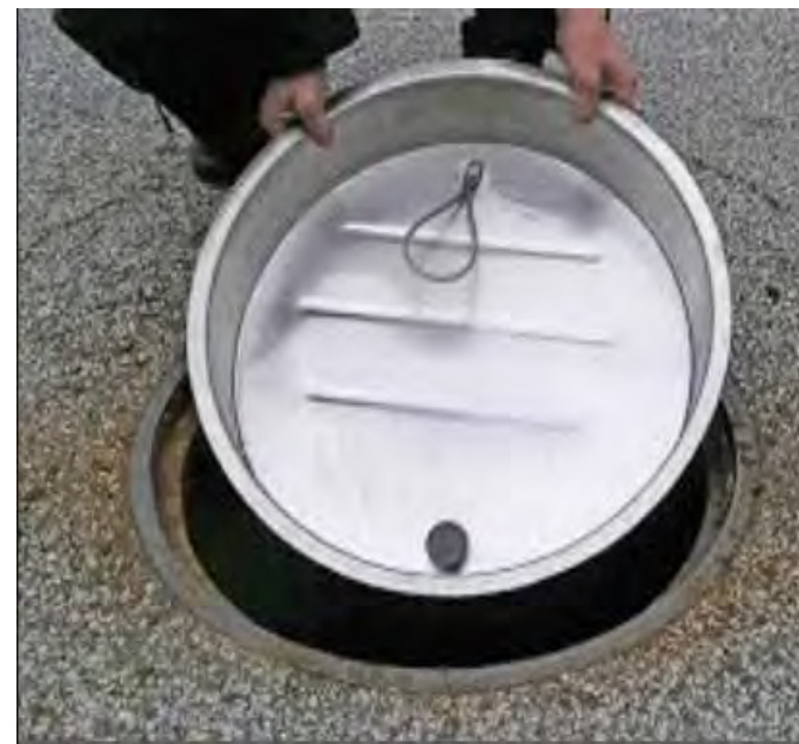
Inflow insert (pan) being installed in a manhole to mitigate surface water entering the sanitary sewer system
